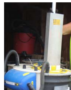
Fluorescent tube crushing at Corral Farm Convenience Site
