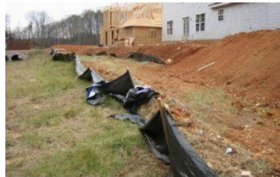
Silt Fence Failure
