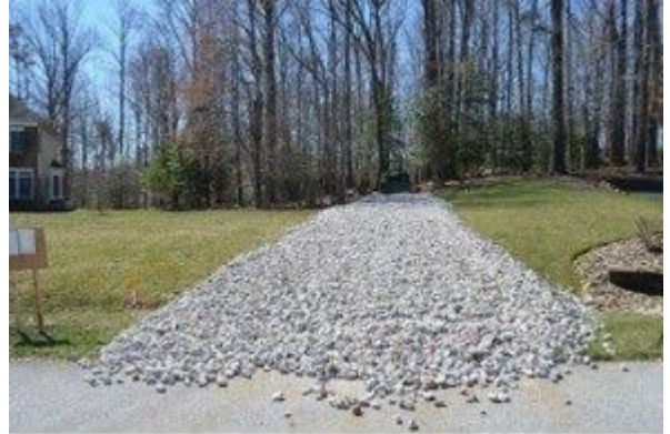
Improperly Maintained Stone Construction Entrance- Stones Dislodged Spilling into Adjoining Roadway
